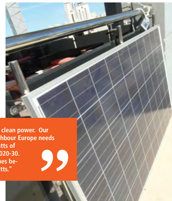
□ Solar panel on hotel in central Tripoli
